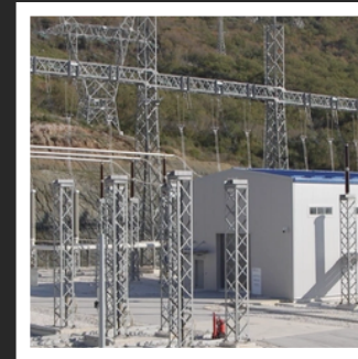
ELECTRICAL SUBSTATION BREZNA
